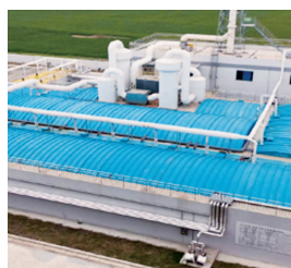
Sewage station of Suzhou Erye
